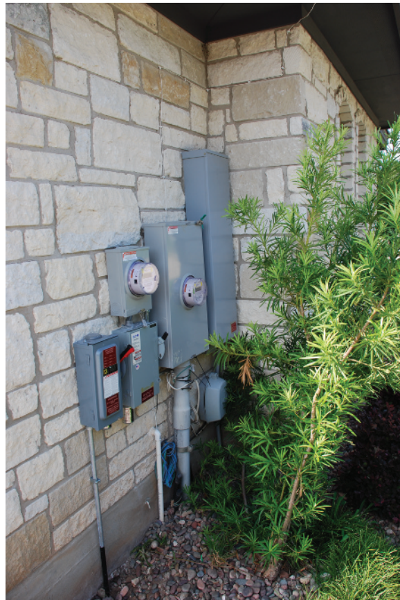
FIGURE OCCUPATIONS 6 One meter records the power supplied by the utility company, and another records the amount of power supplied by the solar panels.
