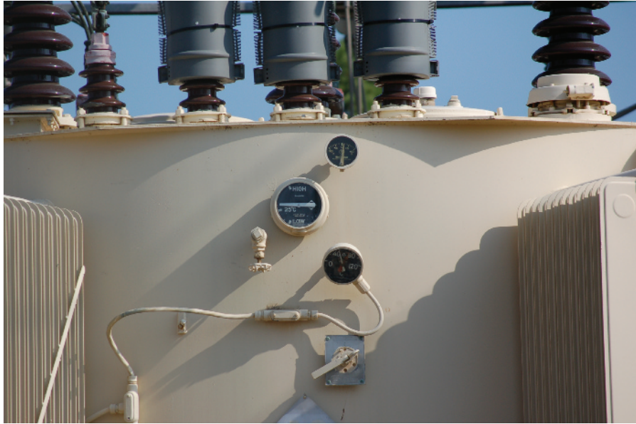
FIGURE 28-4 External gauges used to monitor a sealed transformer.
