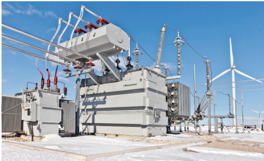
FIGURE 28-3 Pad-mounted transformer. Courtesy of SPX Transformers Solutions, Inc.
