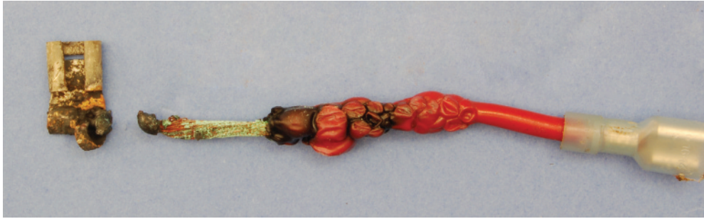
FIGURE S-19 Burned wire caused by a poor connection.
