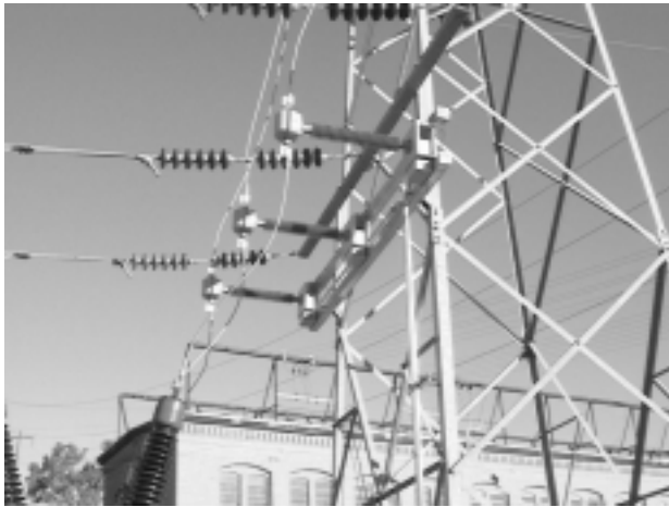
Figure 11-41. 72 kV Magneto-Optic Current Transducers at Substation.
