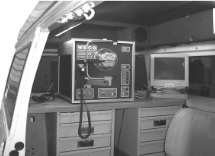
Figure 14-17. Mobile Meter Testing Facility.
